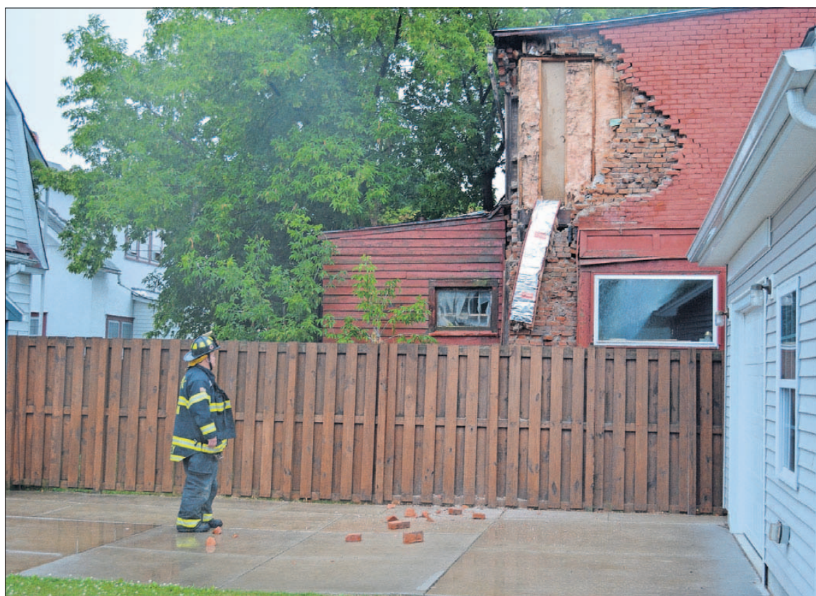
Hornell Fire Department Captain Brian Tingley surveys the damage after a partial wall collapse at 10 Cottage Ave. in the city Monday afternoon. PHOTOS BY RYAN PAPASERGE/THE EVENING TRIBUNE
