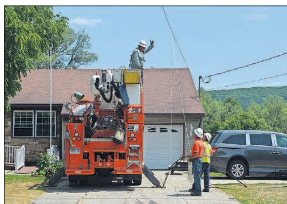
A NYSEG crew works to repair a power line on North Main Street Extension Monday afternoon.
