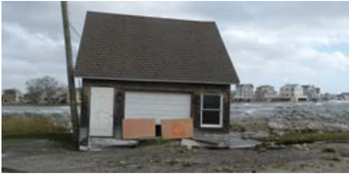
Condemned house in Westbrook, CT after Sandy. © Adam Whelchel/TNC
