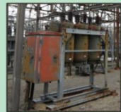
34.5 kV Oil Circuit Breaker
