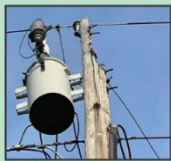
12.5 kV Distribution Pole (w/ Top Rot)
