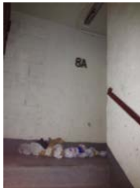
Besides the debris, the light out in this stairwell renders it an especially dangerous landing.
