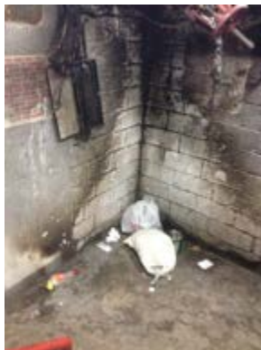
Debris already accumulating near the site of a recent fire in Marble Hill Houses.
