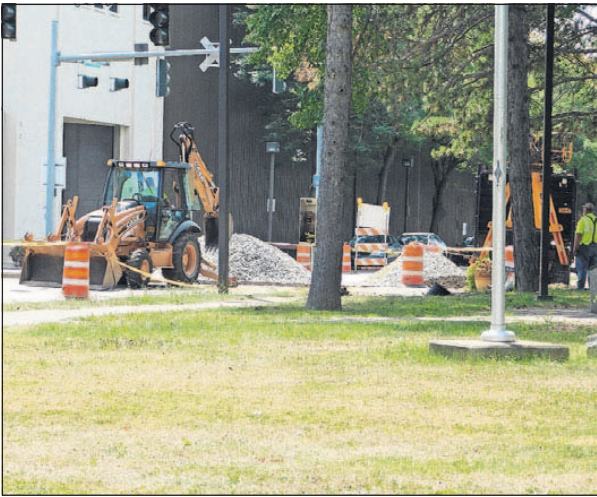
B&H Rail Corporation is replacing the railroad crossing on North Hamilton and West Chemung Street in Painted Post. The crossing is closed to traffic. Painted Post Department of Public Works Superintendent Larry Smith said the railroad informed him the crossing would be completed Thursday or Friday. STEPHEN BORGNA/THE LEADER
