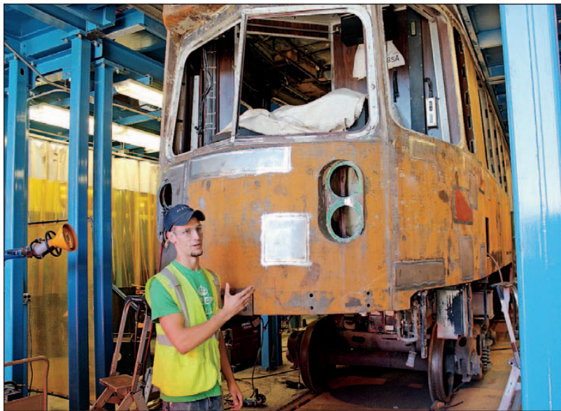
Alstom welder Ben Bennett explains how he and his co-workers patch rusted and smashed bodies of Green Line cars that are 1980s vintage as they roll through the shop. The experience of dealing with older trains has prepared him well for tackling the upcoming Amtrak contract, building high tech designs from scratch. JOHN ANDERSON PHOTO
